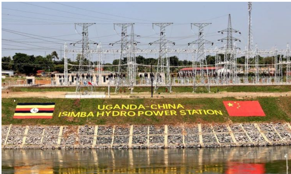
Figure 1-2 Isimba Hydropower Station
